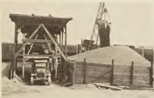
FIGURE 1.—A THREE-COMPARTMENT BIN AND THE EFFECTIVE USE OF PLANKS GREATLY REDUCES THE AMOUNT OF SPACE NECESSARY TO HANDLE TWO SIZES OF AGGREGATE
